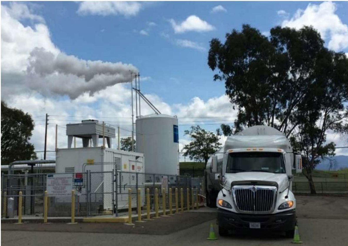
Figure 6.2: Removal of displaced gaseous hydrogen via the chimney of the storage tank during LH 2 delivery. Due to the coldness of the discharged gas, moisture condenses locally from the air and a cloud of fog forms. Source: 13
