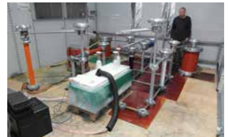
Fig. 3: Three-phase current test with the Combutt system with a voltage of 86.6 kV (effective, phase against phase).
